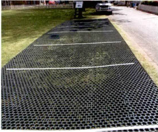
The above image shows the plastic green gridforce system freshly installed, this is within just a few days of installation, no grass has been allowed to grow through the grid force at this stage
